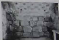
Fig. 103. S. Silvestro in Capua. Foundation wall of north wall of east bay and lower part of superstructure of east bay.
